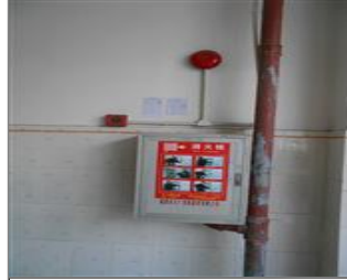
Photo of fire safety equipment fire safety equipment.JPG
